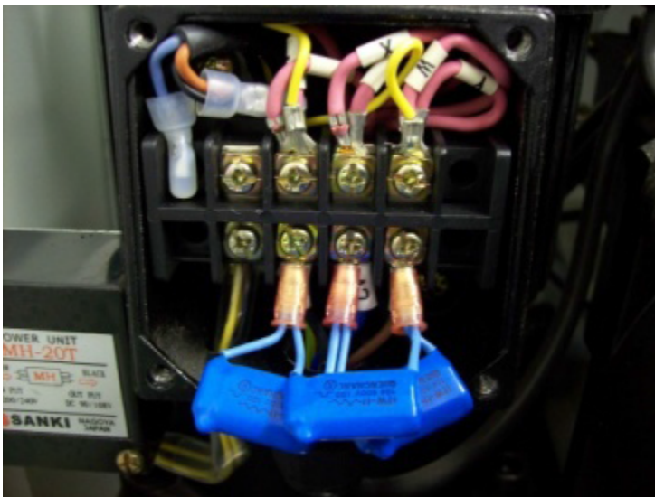
Picture 4: Snubber installed on swing-arm motor
