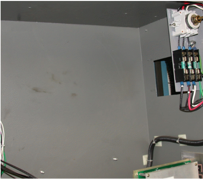
Picture 1: Electrical Cabinet:
